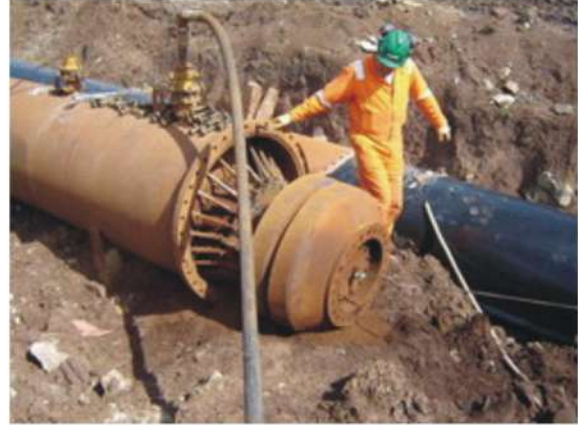
Photo of maintenance oil pipe lines
