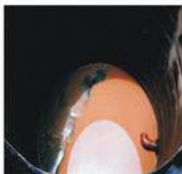
Photo Of sludge in tank bottom
