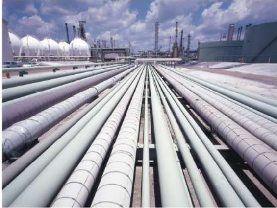
Photo of oil pipe lines
