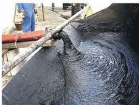
Photo Of sludge coming out of storage tank
